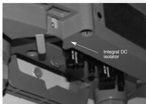
Figure 3-11: DC isolator fitted to Mastervolt Sunmaster Inverter
