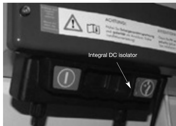
Figure 3-10: DC isolator fitted to SMA Sunny Boy Inverter
